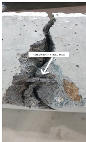
Figure 11. Failure of steel bar.
